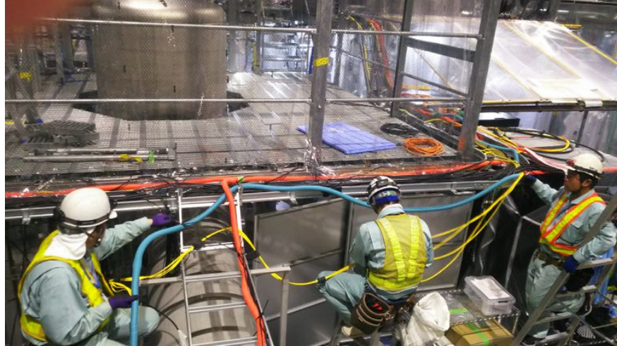
Figure 3: A picture of the fiber installation work around the PR2 chamber in August, 2018. The yellow cables are the optical fibers being inserted into the light blue PF tubing. The black spongy materials are attached to the optical fibers before the insertion.
